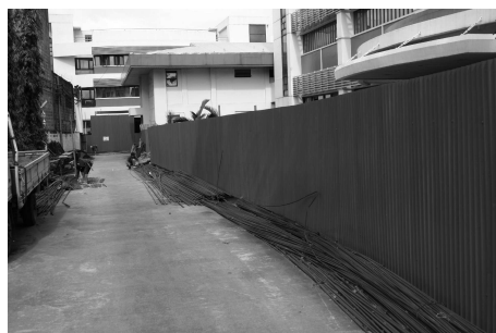
The campus premises have been fenced for the construction activities and safety of the BSOP populace. (December 16, 2005)
